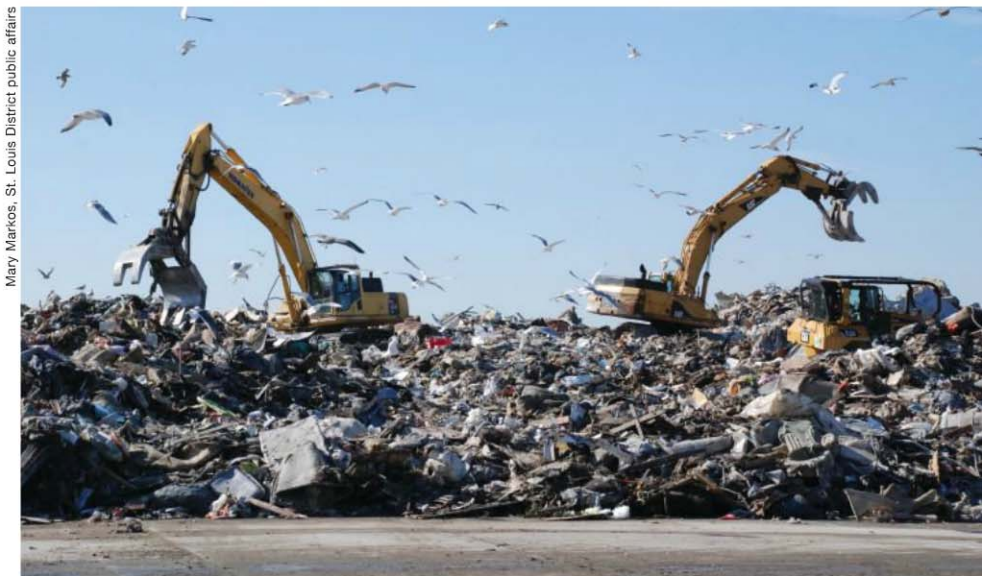
Debris is collected and then loaded onto trucks at Jacob Riis Park in Far Rockaway in Queens, NY, for shipping to landfills.
