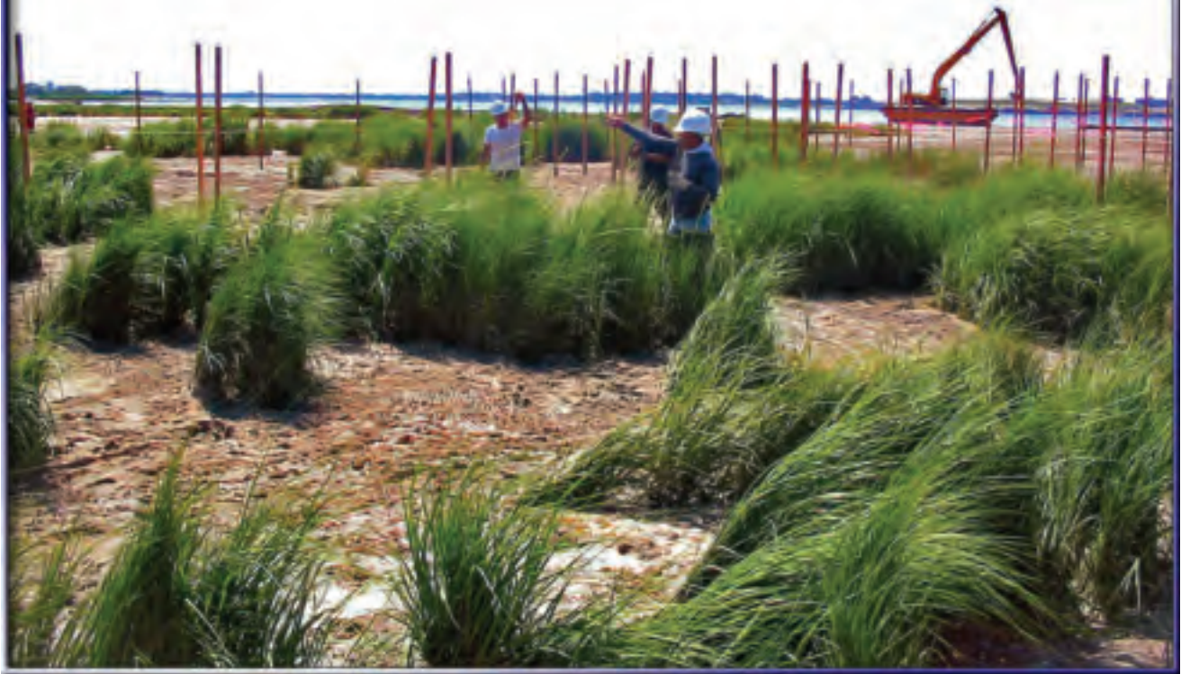
Native grasses being transplanted by hand out of historical marsh, Elders West. Photo courtesy Galvin Brothers, Inc.
