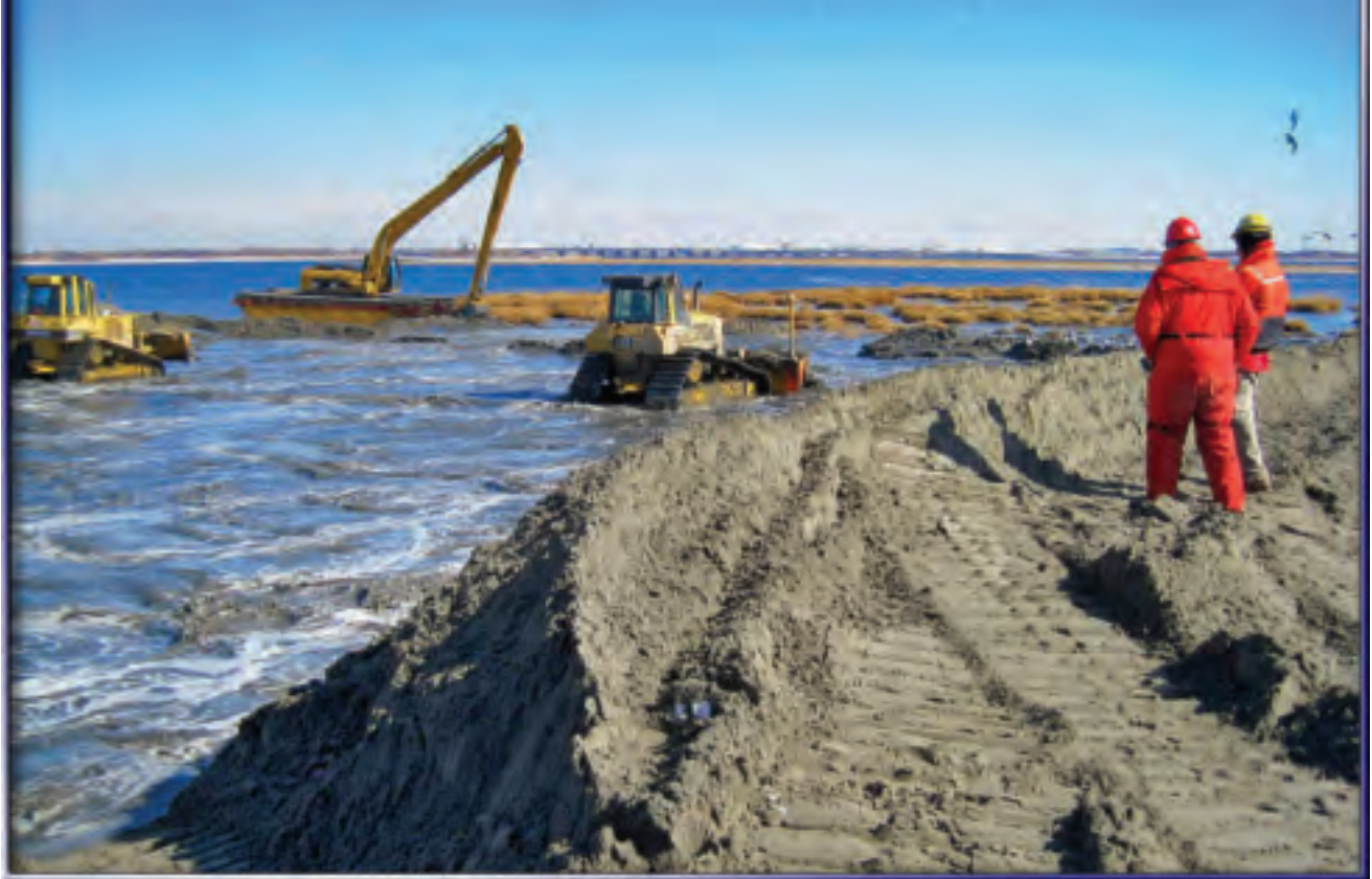
Dredged sand being placed and graded on Elders West. Photo courtesy USACE, New York District.
