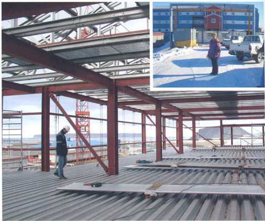
Contractors inspect the installation of flooring system metal decking. Inset: JoAnne Castagna, Technical Writer, USACE, New York District, stands in front of the dormitory in April 2006.
