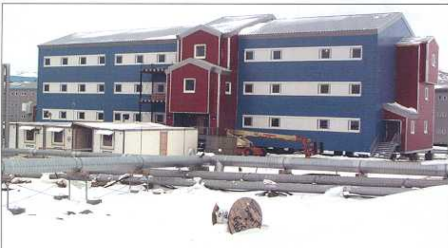
Due to harsh Arctic conditions, outside construction is limited to summer and fall months.
