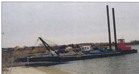
Inner Space Services used the 14 x 12-inch dredge Mardi Gras to pump 60,000 cubic yards of material from the Long Island Intracoastal Waterway a maximum distance of 7500 feet to East Inlet Island. Courtesy Inner Space.
