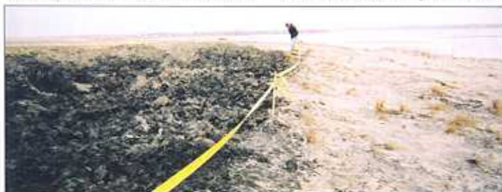
John Riffey, III, B+B field engineer, marks off an area that was left in a tilled state for further drying. Photo courtesy B+B Dredging.
